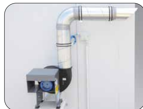
Ex-proof exhaust fan incl. exhaust air monitoring
