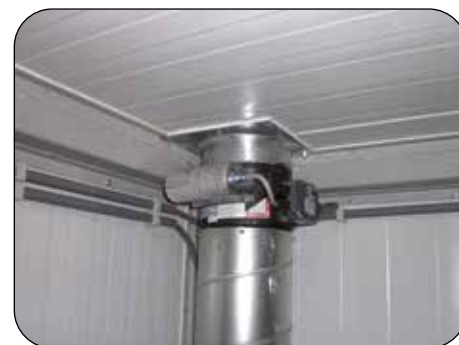
Air exhaust duct with K-90 shut-off device
