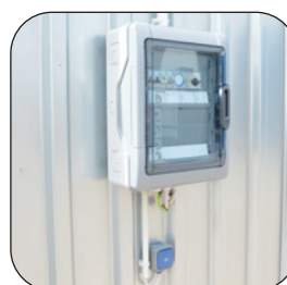
Switch box, Article no. H63-9007-A
