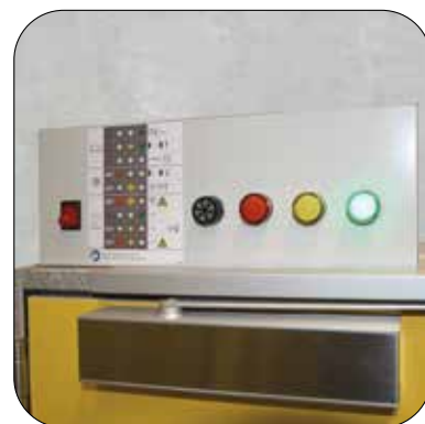
Control unit with fire detection
