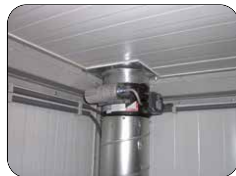
Air exhaust duct with K-90 shut-off device
